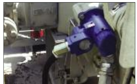
T20 installed on a CAT G3306 compressor.
